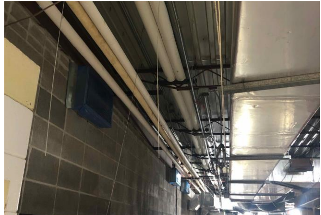
Mech. system above ceiling be re-supported
