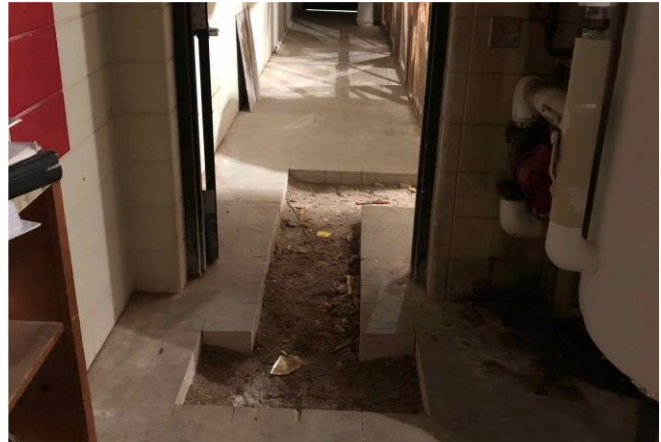
Underground Plumbing in Lower Level.
