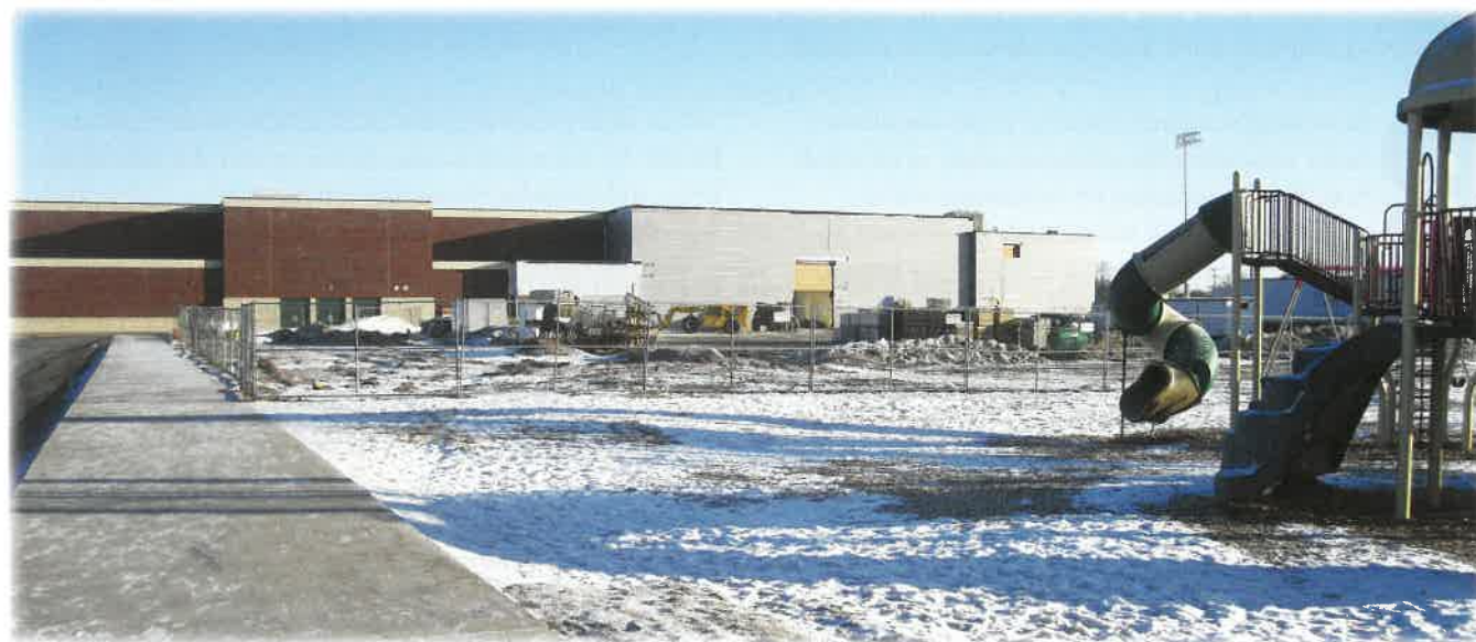
Setting up areas of construction that are fenced off, secure, and only accessible by trained construction personnel is a critical component of any safety management plan.
